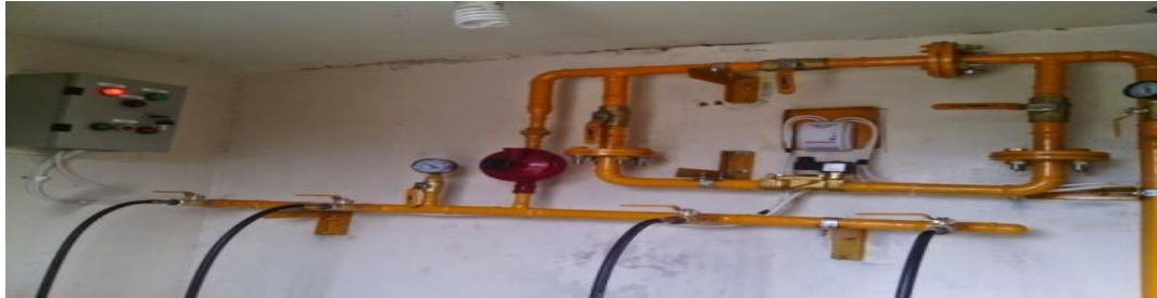
Instalasi gas & panel kontrol
